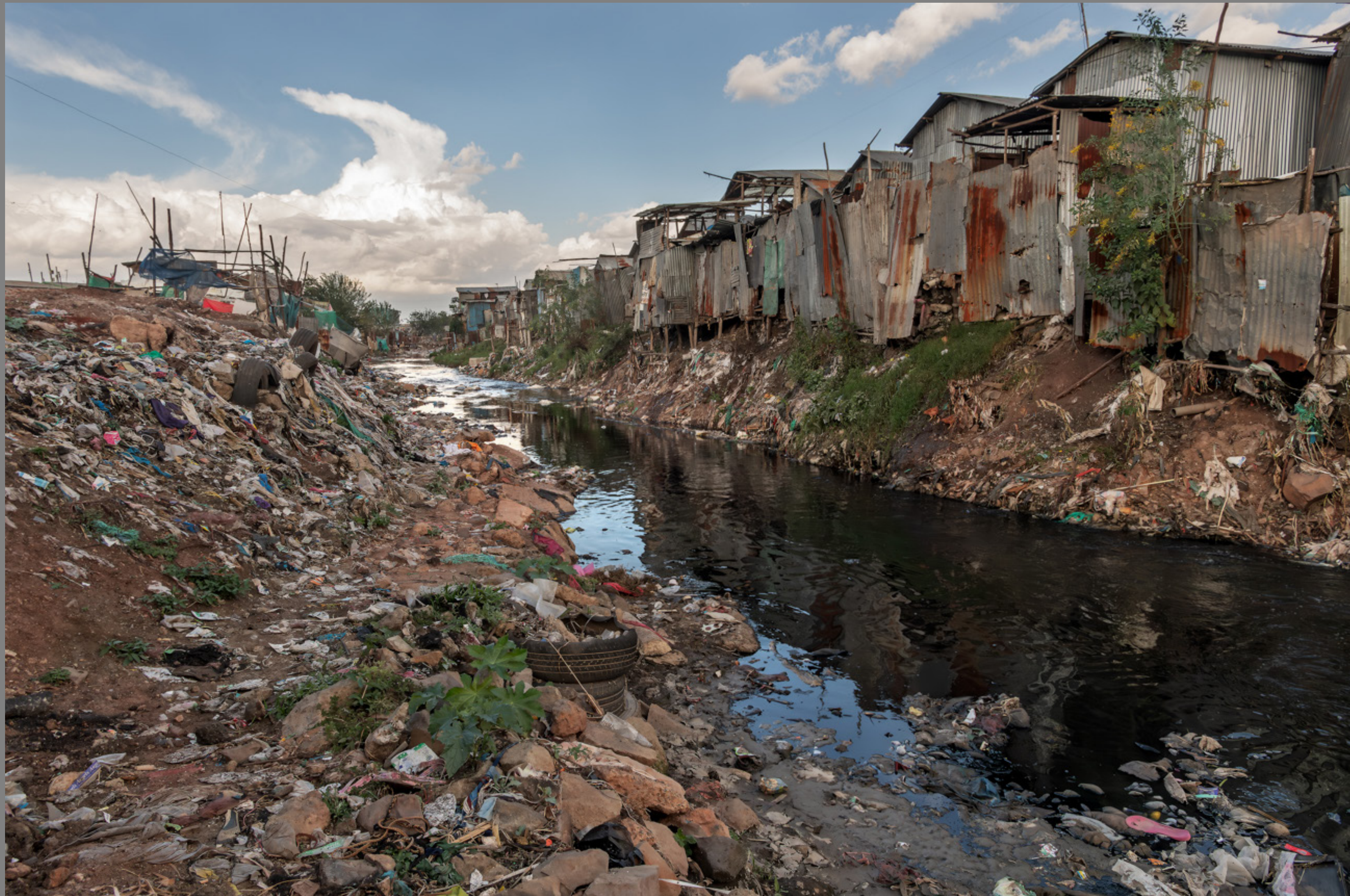
Following the overflowing of the river that runs through Lunga Lunga, due to the floods that hit Kenya in the spring of 2024, the government ordered the demolition of all houses built along its banks. A precautionary measure to avoid further casualties in the event of new floods. However, it has effectively deprived thousands of the slum's inhabitants of a roof over their heads, who have been offered no alternative solution to simple forced eviction.
